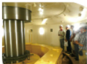
Underground Electric Generation Facility
